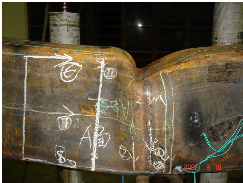
Fig. 7 Picture of the plastic deformation on the crossbeam
