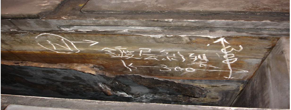
Figure 3. Close view of outward appearance of damage mold in pouring gate
