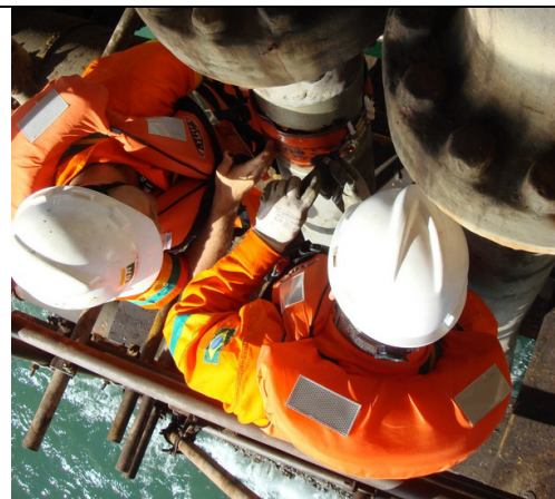
Figure 8 – Installation close to splash-zone on an un-cased offshore riser.
