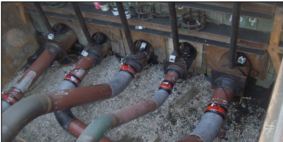
Figure 5 – Several gPIMS ® sensors installed on cased road crossing pipes.
