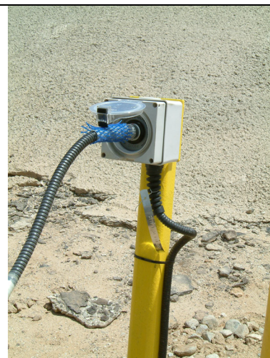
Figure 2b) – Connection box
