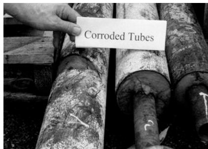
Fig. 2. Samples of heating tube take out from the network due to heavily corrosion level
